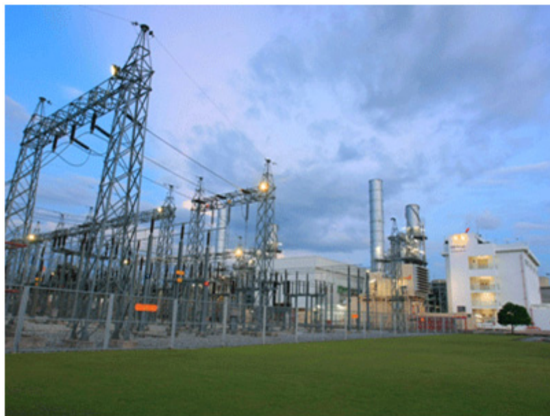
Figure 6. Chana power plant
