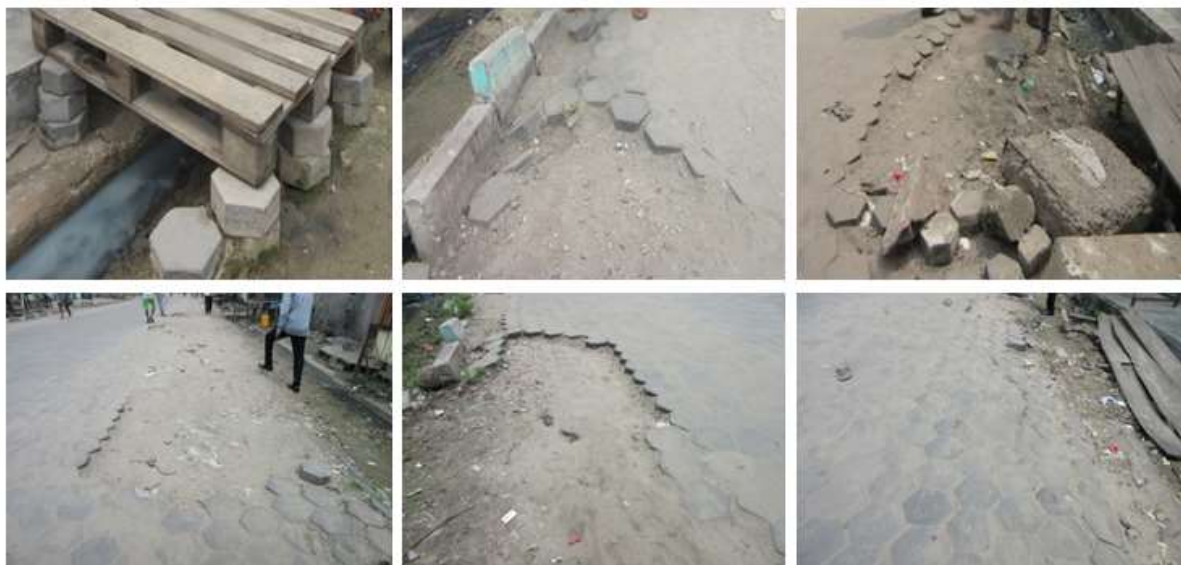
Fig. 5. View of dilapidation of the framing edges
