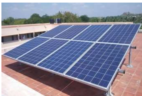
Fig. 5. Solar roof top PV panel system
