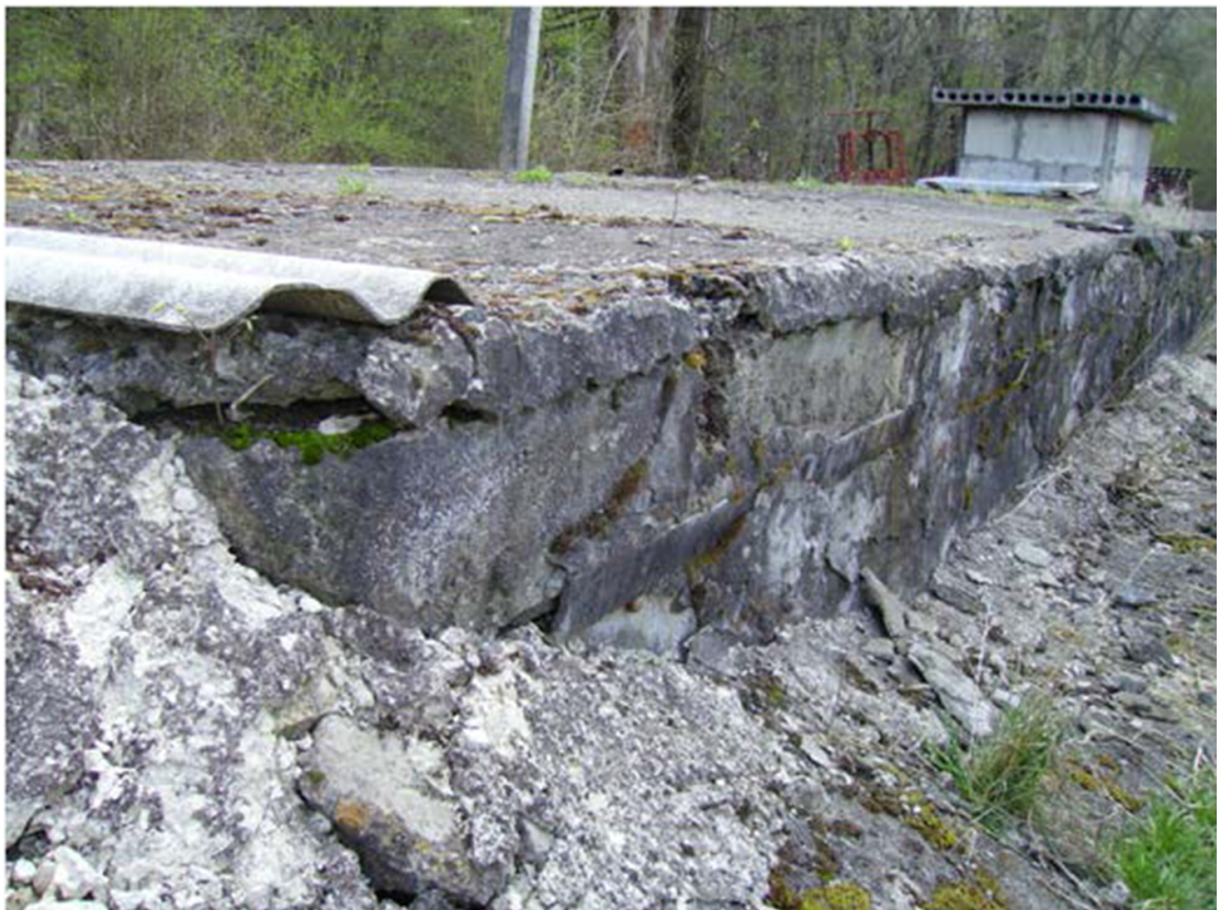
Figure 3. Condition of the facility showing evidence of weathering of the concrete structures (Anton 2017). Reproduced with permission from Anton (2017).
