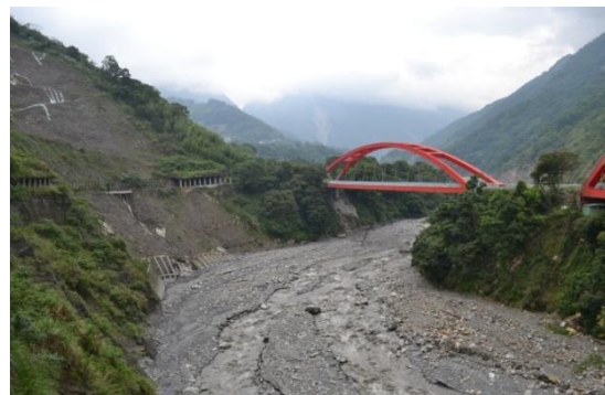
Fig. 5. The Dongpu Moon Bridge (The figure on the left is the original tribes outside of the road, as the attacked of earthquake and typhoons, road side the hillside collapses, the tunnel collapsed and fall into river.)
