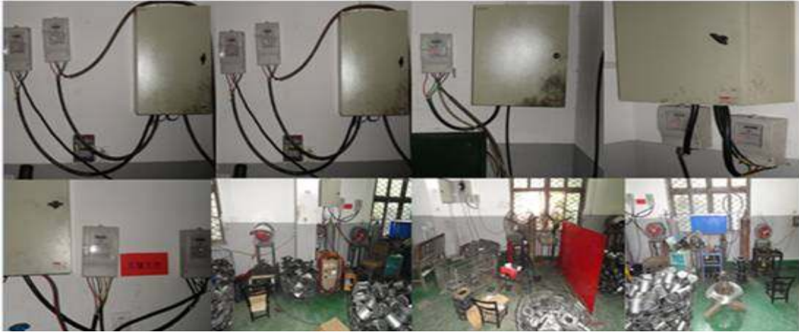
Fig. 2. Meters (kWh) for power consumption monitoring
