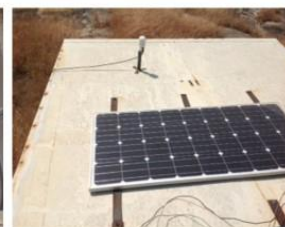
GPS and Solar Panels
