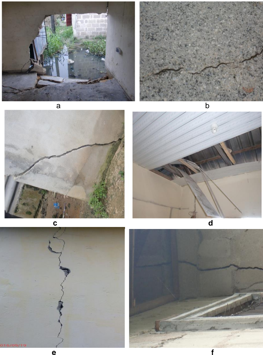
Fig. 7. (a) Collapsed building at Igbogene, (b) Crack and subsidence on a coal tarred road at Igbogene, Bayelsa State (2016), (c) Building almost collapsing at Ishiayi, Rivers State (2016), (d) Building showing caved-in ceiling in one of the communities, (e) Cracked wall from impact of tremor in Kwoi Kaduna state 2016, (f) Building with cracked wall at Mbiama, Rivers State (2016)
