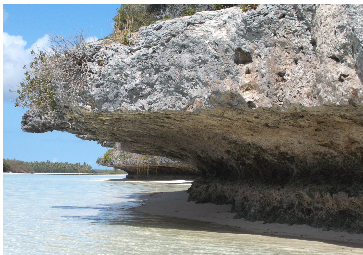
Figure 33. The present under-cut notch is quite impressive, too.
