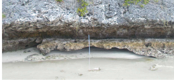
Figure 34. The present under-cut notch ends in a horizontal bench located 70 cm above the presently active under-cut and cave erosion at HTL.
